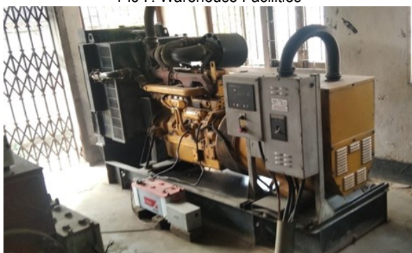
Pic 9: Standby Power Generator Facilities
