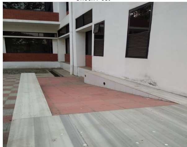
Pic 25: Ramp Facilities for Disable Passengers
